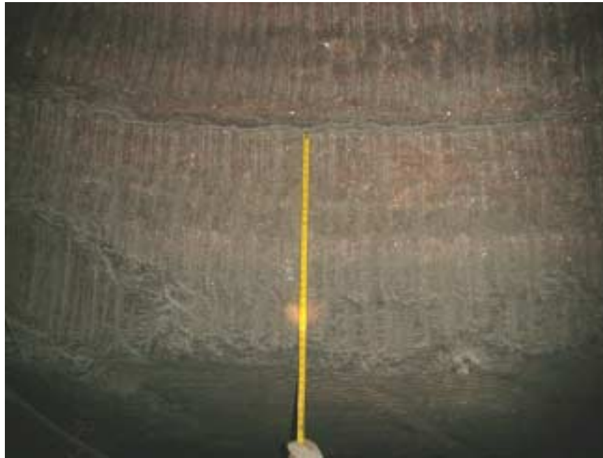
Figure 7: Photo of observed fracture in brow along Main 5 access drift.
